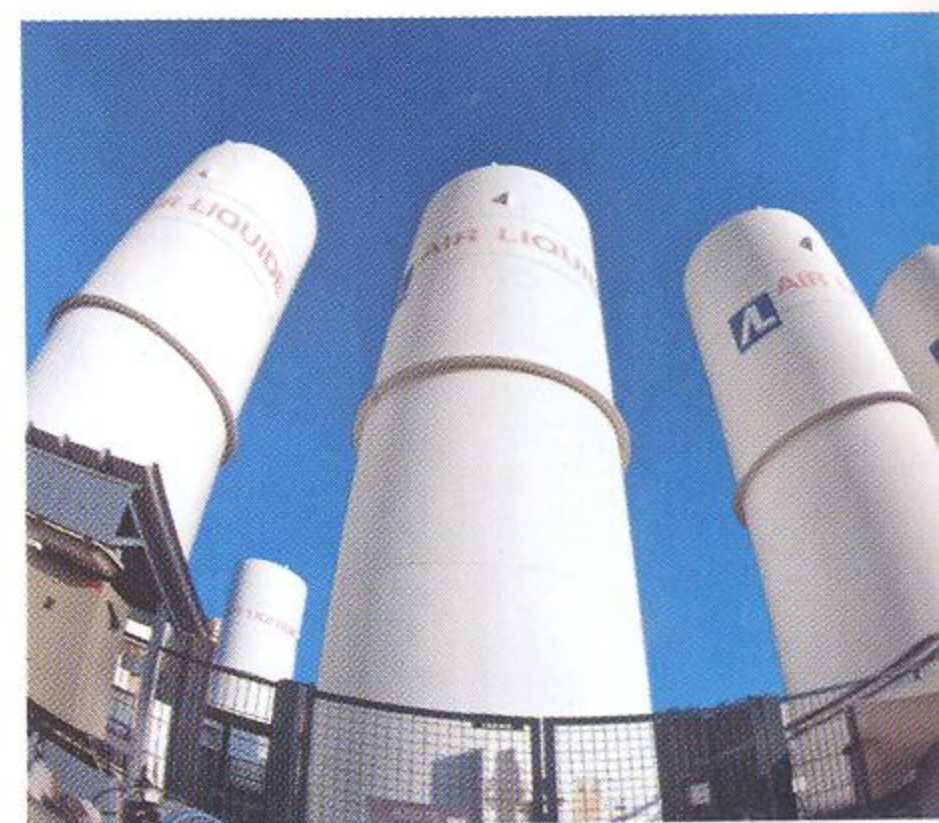
Serbatoi Air Liquide
